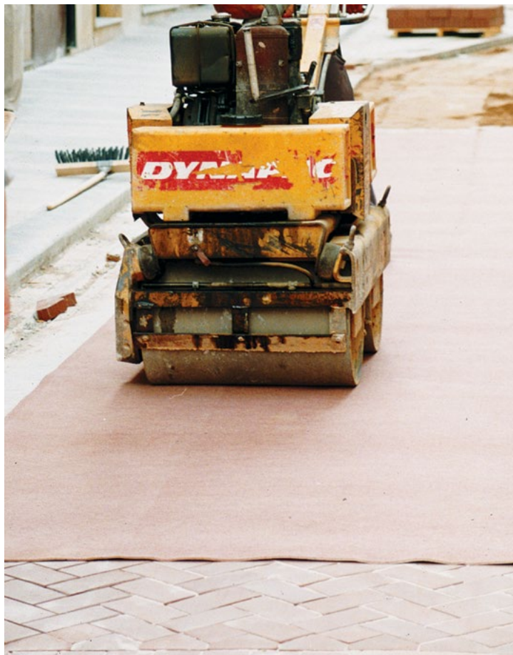
Compacting pavers. Use vibrators with rubber bases, or spread out a blanket as shown in the photo to avoid chipping.
